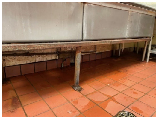
Rusted Kitchen Equipment
